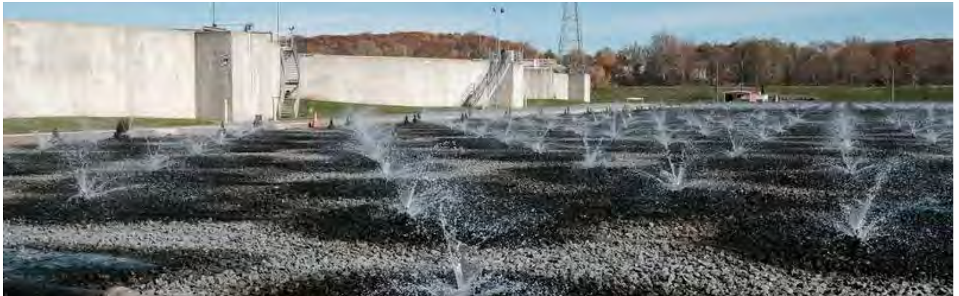
Kline's Island Wastewater Treatment Plant (Image Credit: The Morning Call)
